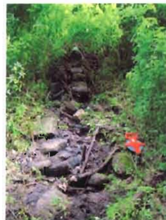
6 - PVC Outfall Pipe
